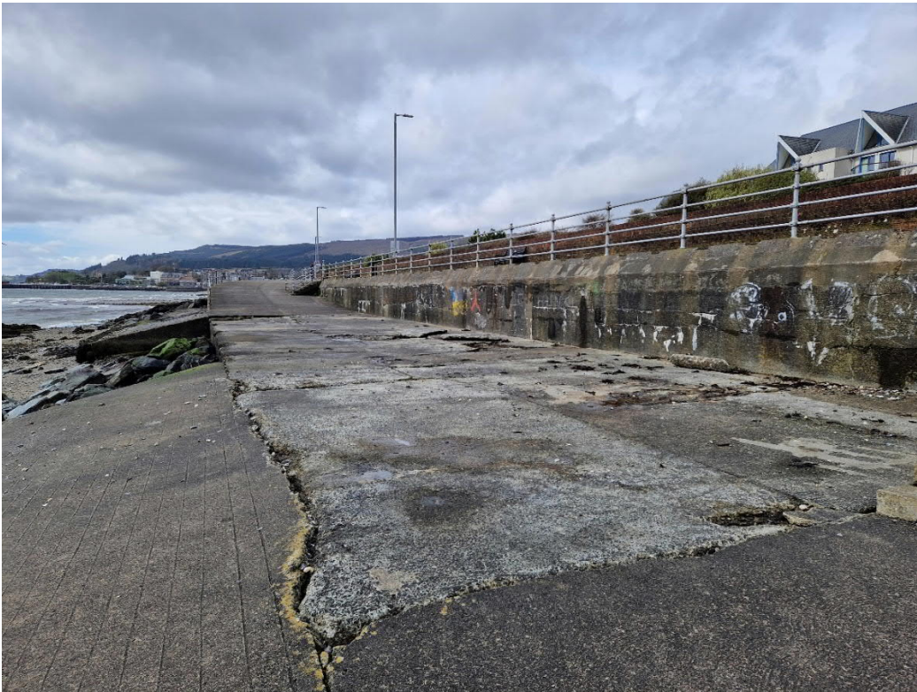
Figure B.3: View of broken deck slabs at parking area, joint with head of slipway
